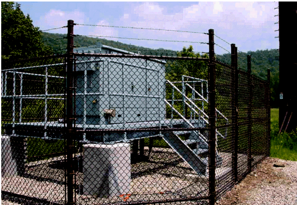
FIGURE 3-4 TYPICAL OUTDOOR ENCLOSURE CABINET ON RAISED PLATFORM
